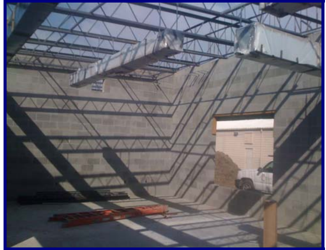
HVAC Ductwork Installed with Ends Protected
