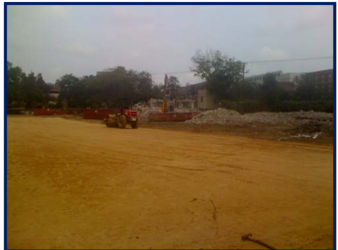
North Wing Building Pad to Grade With South Wing Demolition Near Complete
