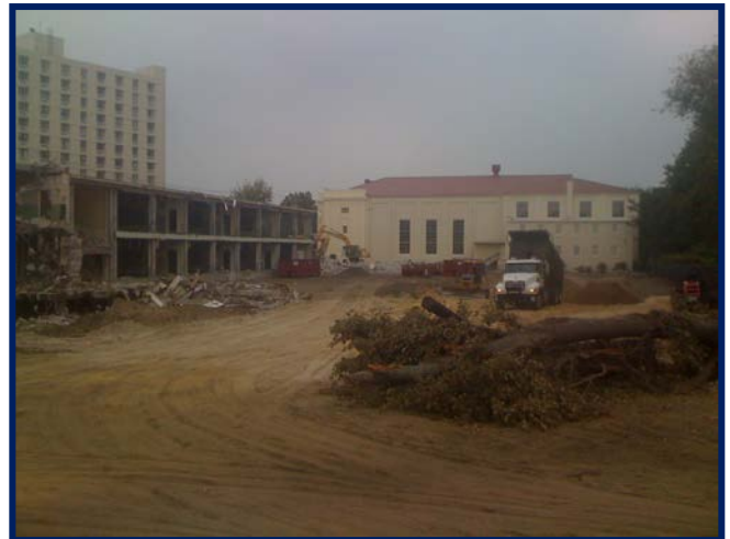
South Wing Demolition in Progress with Simultaneous Installation of Bldg. Pad Material
