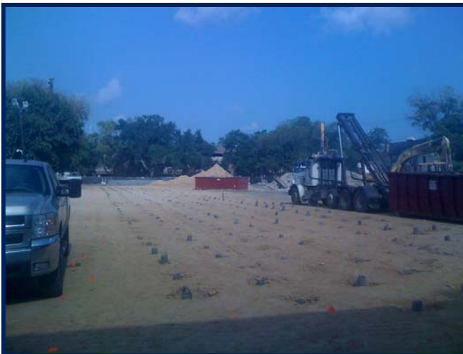
View of Completed Earthquake Drains Installed at North Area of New Building Pad
