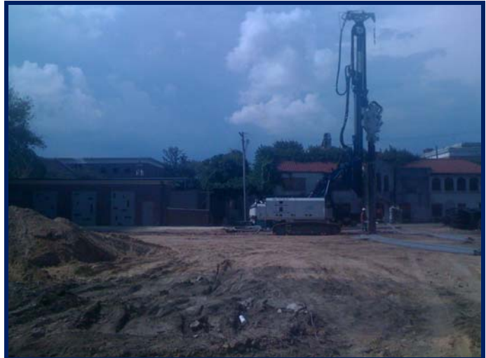
Earthquake Drain Installation Rig at Cafeteria - Multipurpose Area of the New Building
