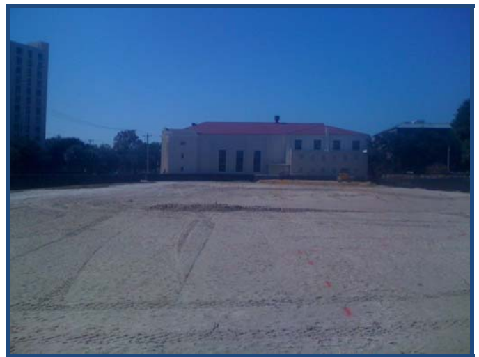
View of Completed Site with Final Install of Fill Material Underway to Complete Contract Work
