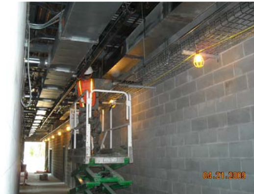
Duct Work Area B
